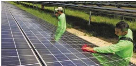
Thailand's Korat 1 solar power station, owned by new IFC client Solar Power Co.
