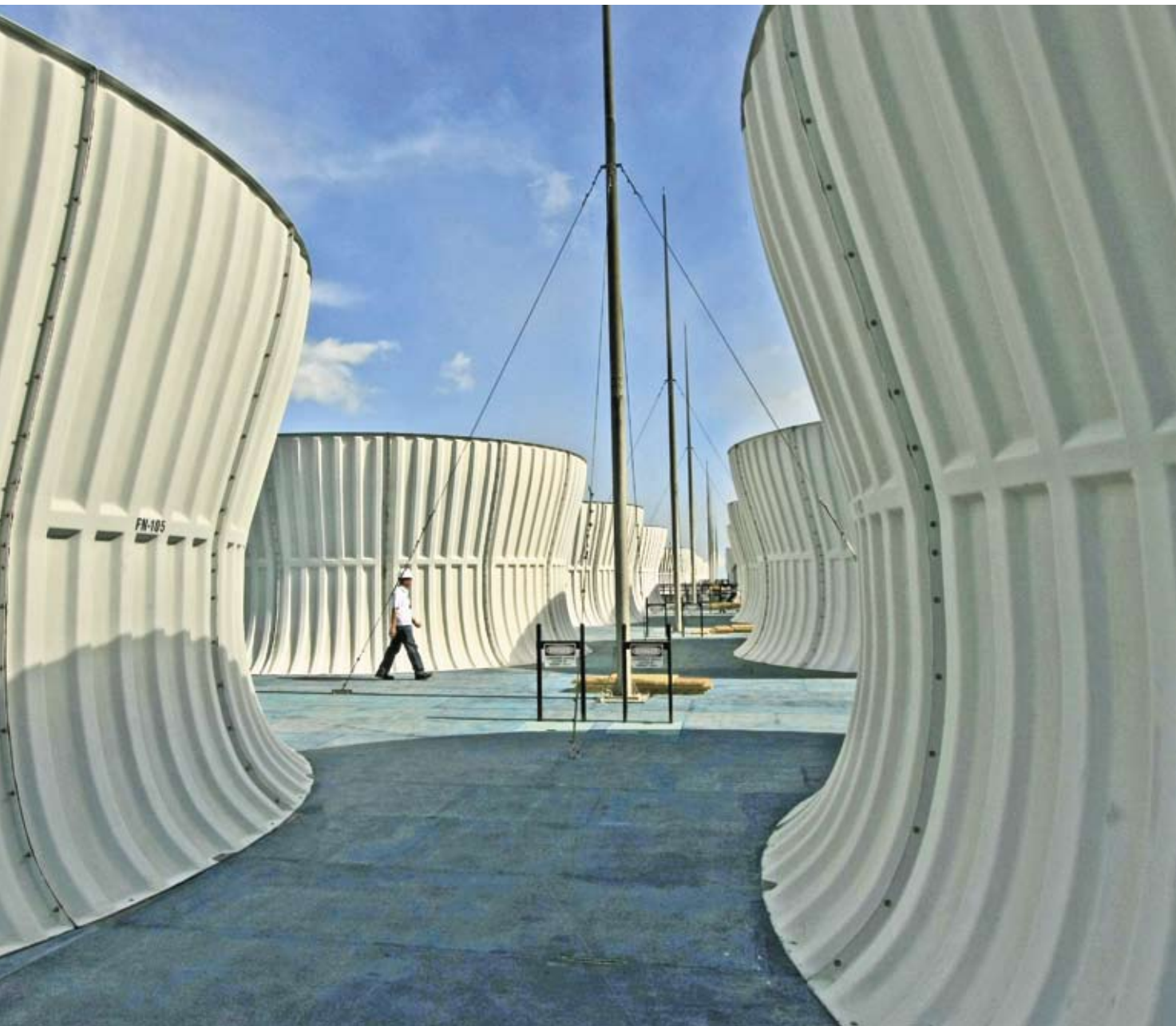
Advanced cooling towers are just part of the impressive technology at the Philippine geothermal plants owned by EDC, a key player in this important form of renewable energy.
